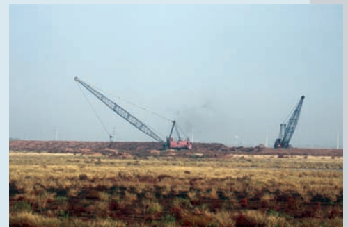
Pipeline construction observed near resting shorebird areas at Bryan Beach Freeport, TX.
